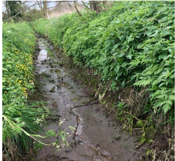
The silted-up drainage ditch before Felbeck Trust volunteers got involved
